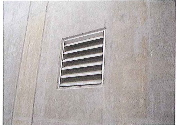
Existing Louver in Generator Room (new louver in Storage Room will be similar)
