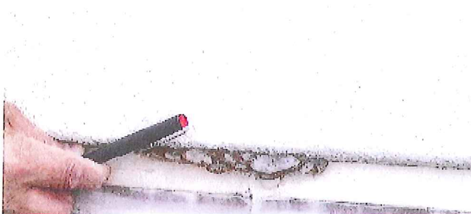
Example of damage to EFIS due to water penetration.
